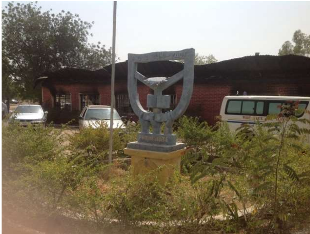
A section of the school burnt down
